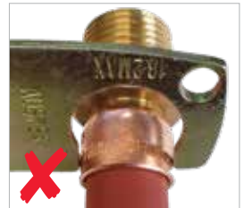
Fitting has been under crimped
