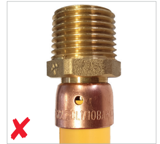
Witness hole not completely filled
