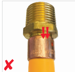
Fitting has been double crimped
