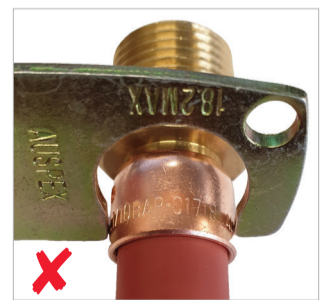
Fitting has been under crimped
