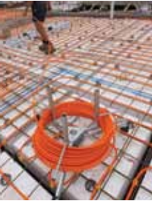
Using the decoiler
